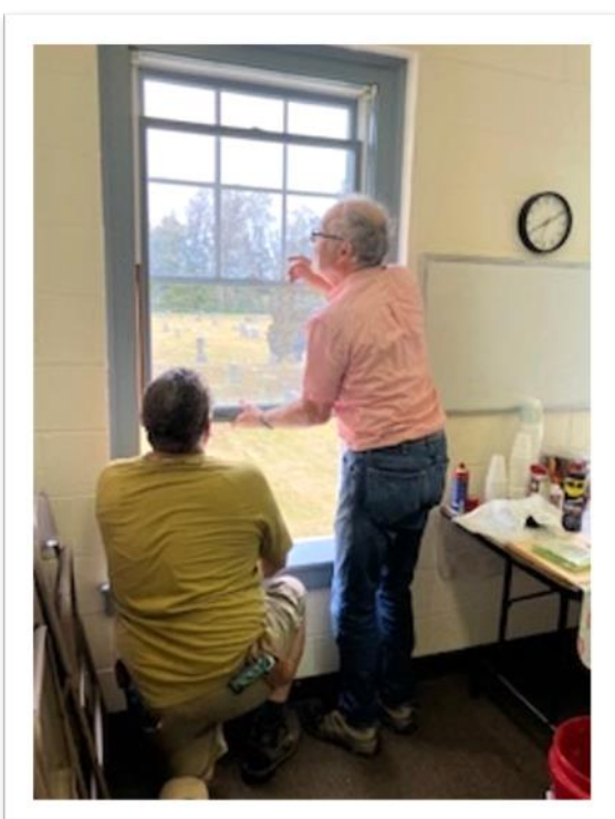
Buildings and Grounds Committee work by Paul Saunders and Rusty Schneider consisted of replacing windows in the second floor of the Godwin Building.
